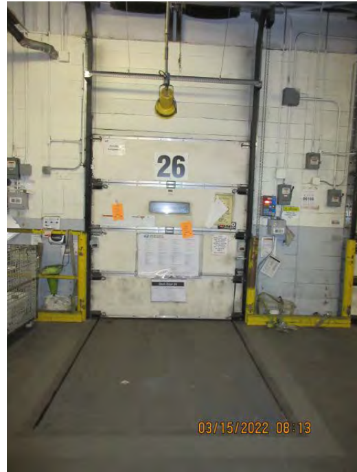
DOOR 26 Install Kelley Dock Communication System
