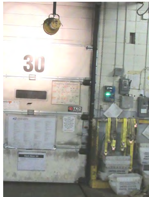
Existing Red/Green Light Controls, Right side of DOOR 30
