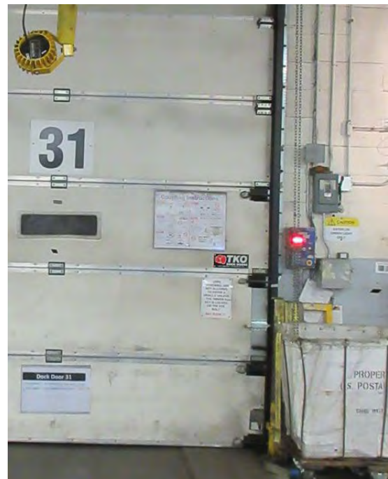
Existing Red/Green Light Controls, Right side of DOOR 31
