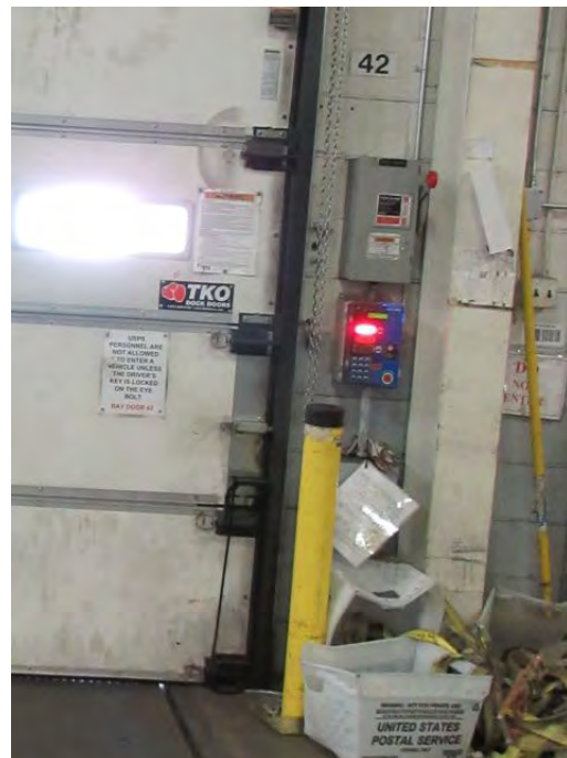
Existing Red/Green Light Controls, Right side of DOOR 42
