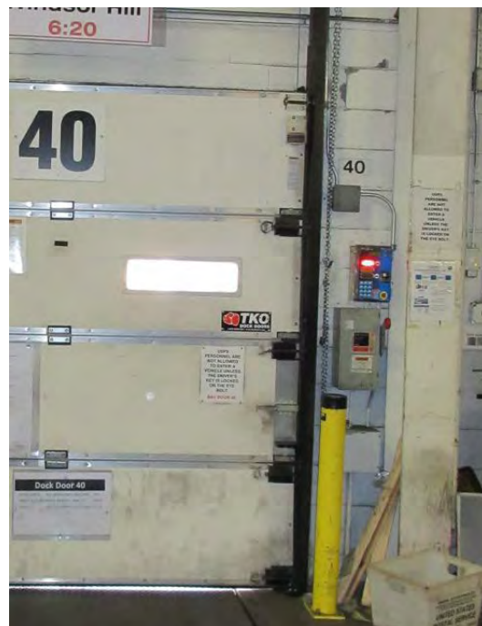
Existing Red/Green Light Controls, Right side of DOOR 40
