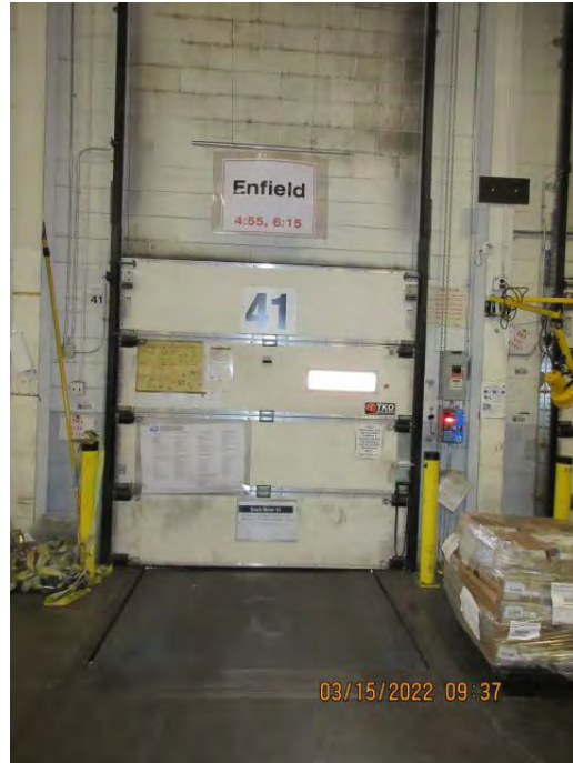
DOOR 41 Install Kelley Dock Communication System
