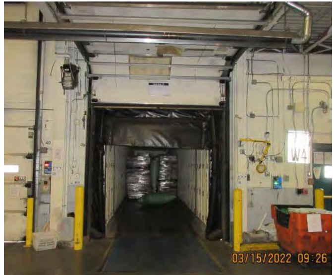
DOOR 39 Install Kelley Dock Communication System
