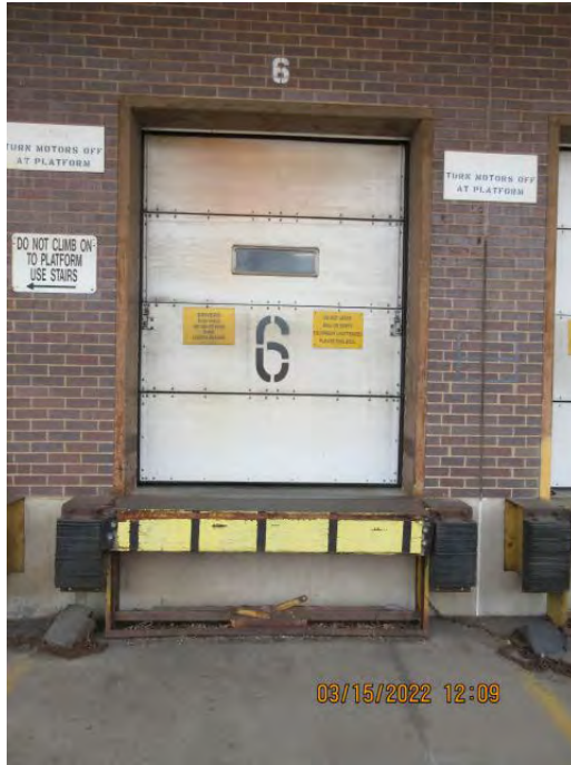
DOOR 6 Install Kelley Dock Communication System
