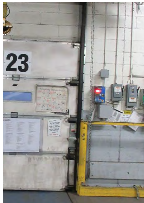
Existing Red/Green Light Controls, Right side of DOOR 23
