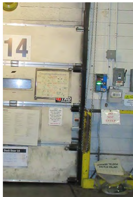
Existing Red/Green Light Controls, Right side of DOOR 14
