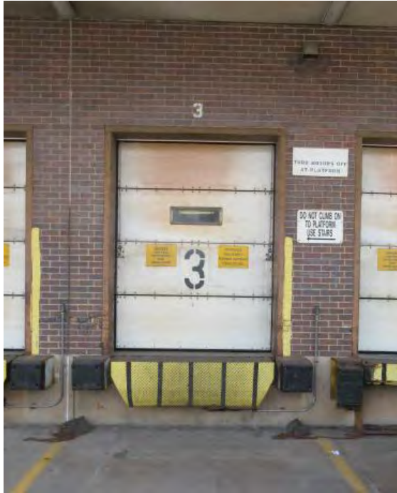
DOOR 3 Install Kelley Dock Communication System
