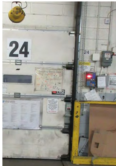
Existing Red/Green Light Controls, Right side of DOOR 24
