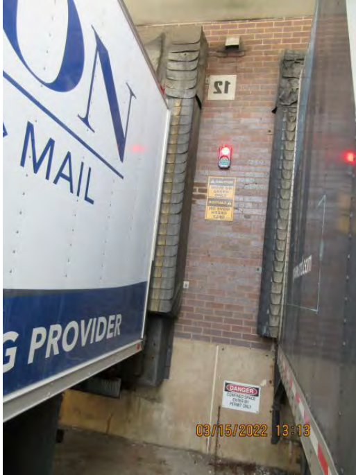
DOOR 12 Install Star 4 Truck Restraint W/ Cantilever Mounting Bracket
