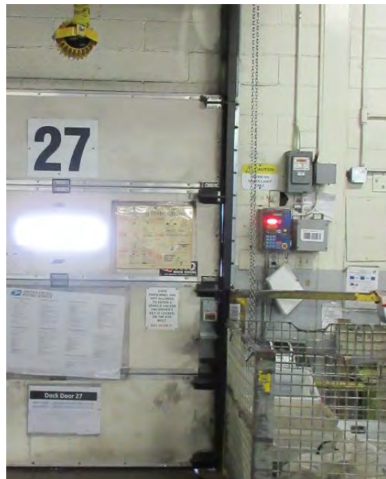
Existing Red/Green Light Controls, Right side of DOOR 27
