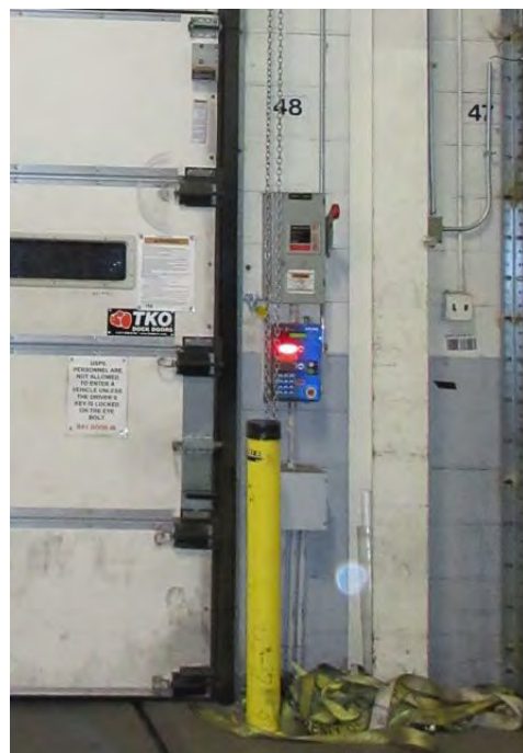
Existing Red/Green Light Controls, Right side of DOOR 48
