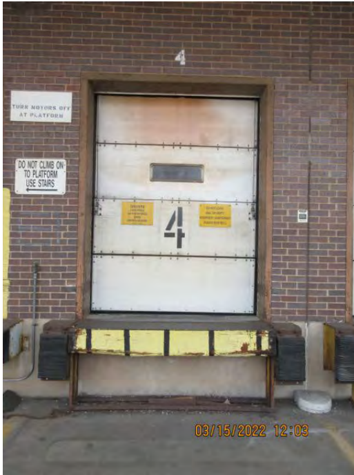
DOOR 4 Install Kelley Dock Communication System
