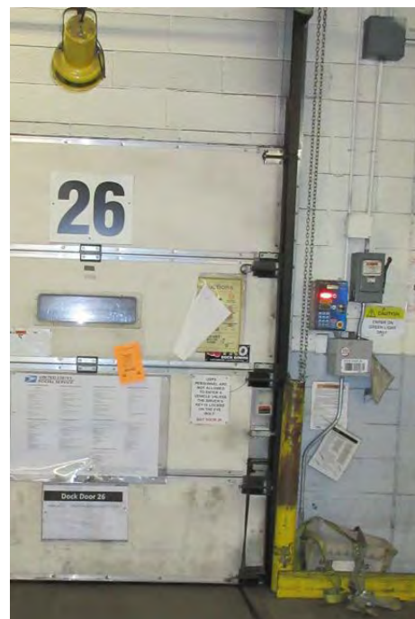
Existing Red/Green Light Controls, Right side of DOOR 26
