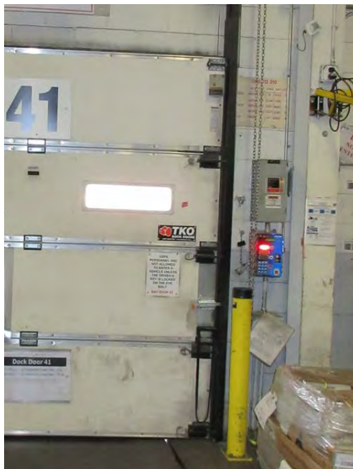
Existing Red/Green Light Controls, Right side of DOOR 41
