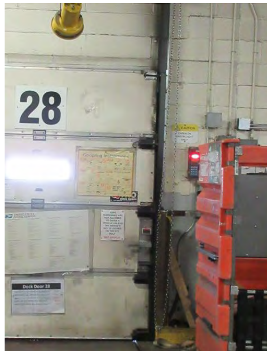
Existing Red/Green Light Controls, Right side of DOOR 28
