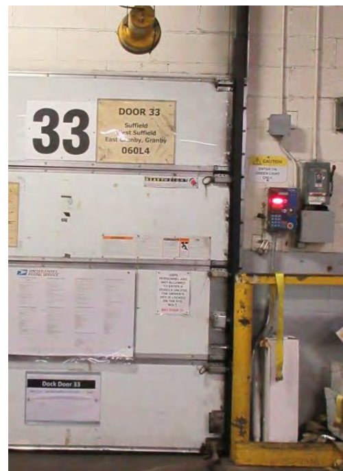
Existing Red/Green Light Controls, Right side of DOOR 33
