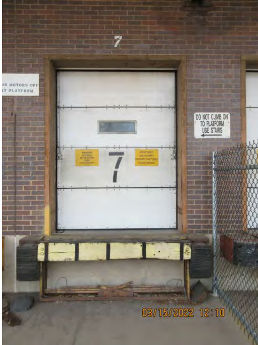
DOOR 7 Install Kelley Dock Communication System
