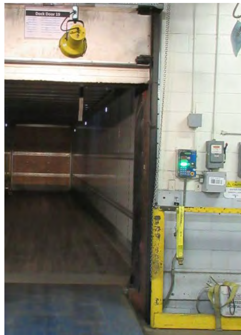
Existing Red/Green Light Controls, Right side of DOOR 19
