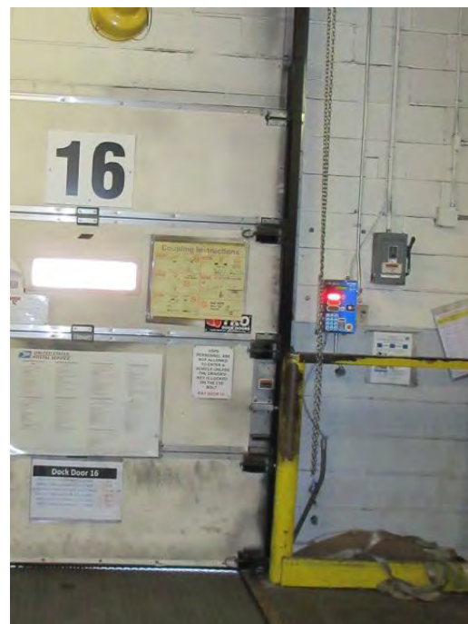
Existing Red/Green Light Controls, Right side of DOOR 16
