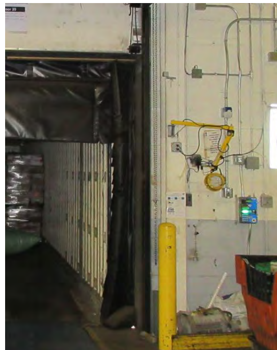
Existing Red/Green Light Controls, Right side of DOOR 39
