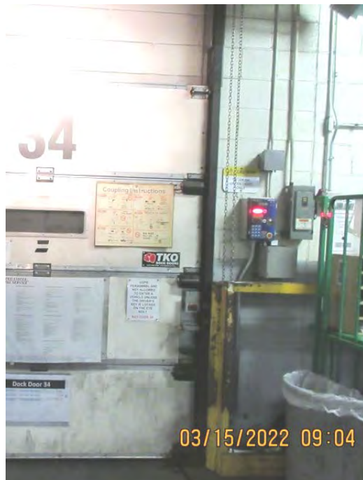
Existing Red/Green Light Controls, Right side of DOOR 34
